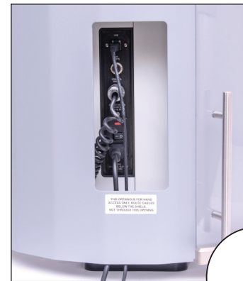
Fig. 3 Proper cable routing
